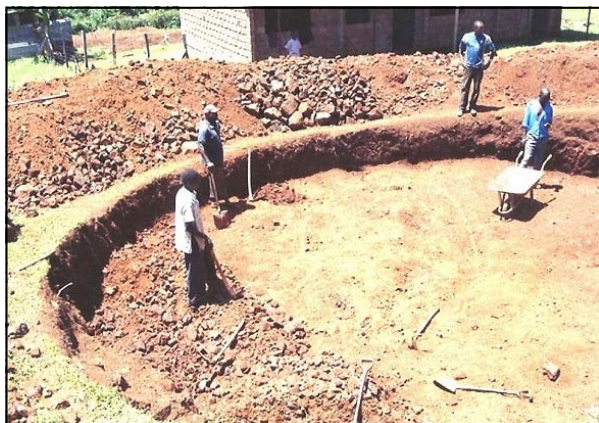
Despite drought, Nyakome School for the Deaf begins construction on their water tank
