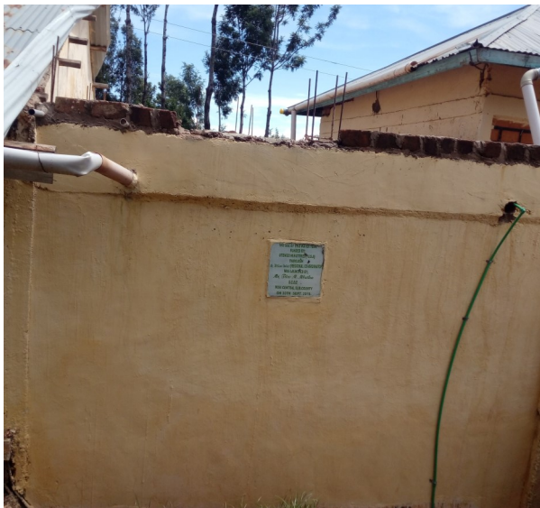
New 66,000-gallon, in-ground water tank at Nyamware
